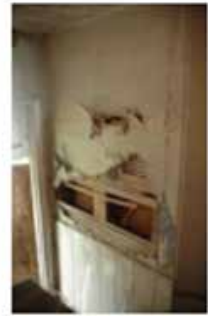
broken lath and plaster
