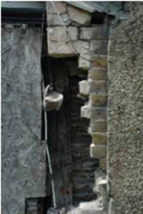
original rear door, internal studding and collapsing brick with render over
